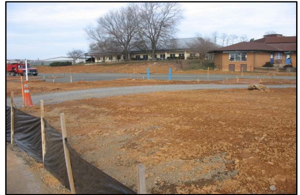
Building pad prior to footings or masonry, existing school buildings in the background
